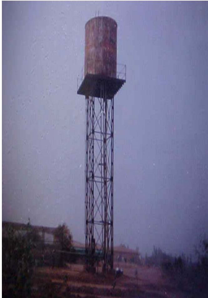
Plate (3.1): The tank
